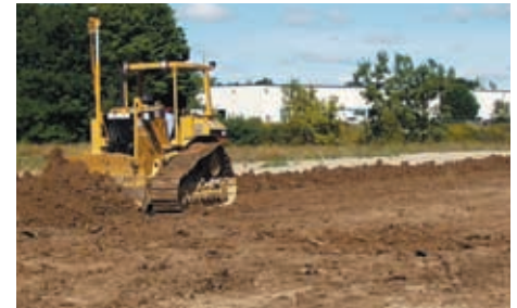
Accurate Grading with auto elevation control for land leveling, sports fields, or parking lots.
